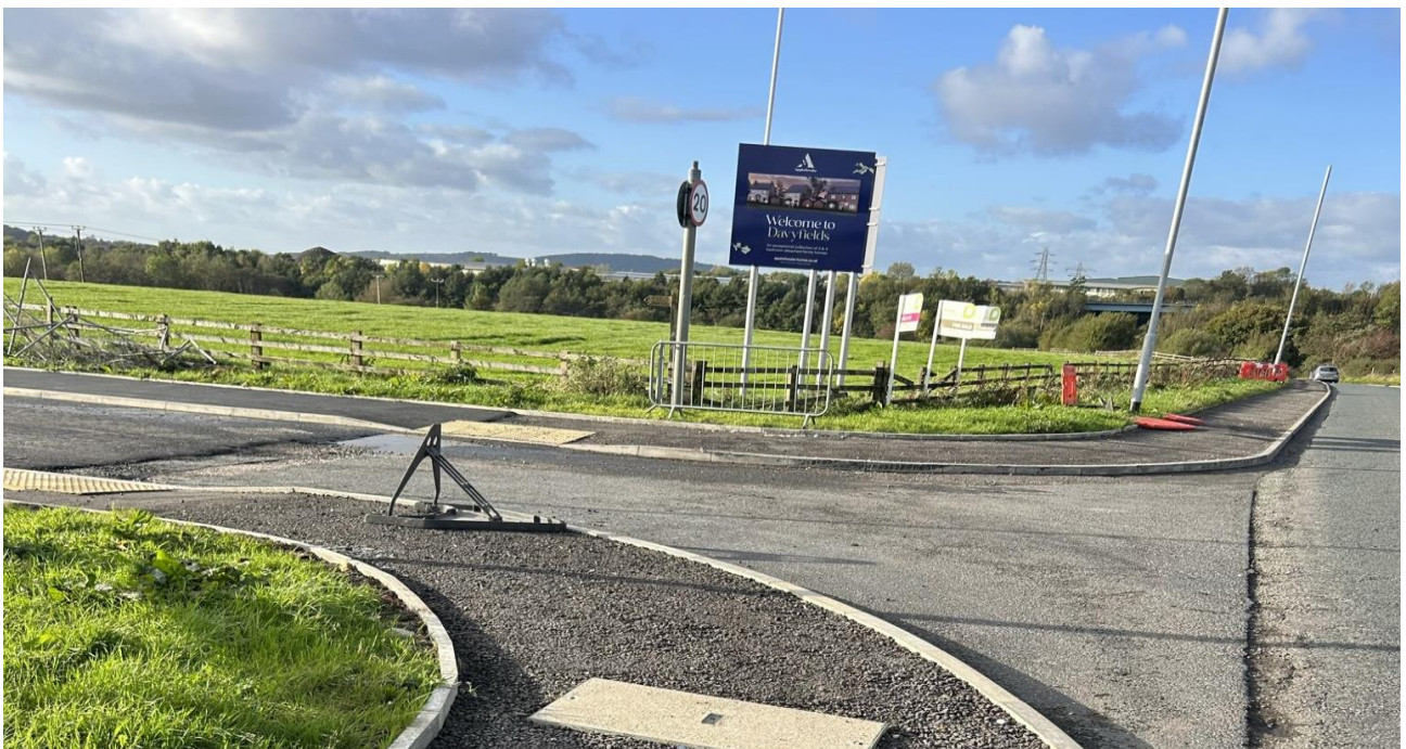
A new footway has been created as part of s278 works for the Applethwaite Homes development at Davyfield Farm, Eccleshill
