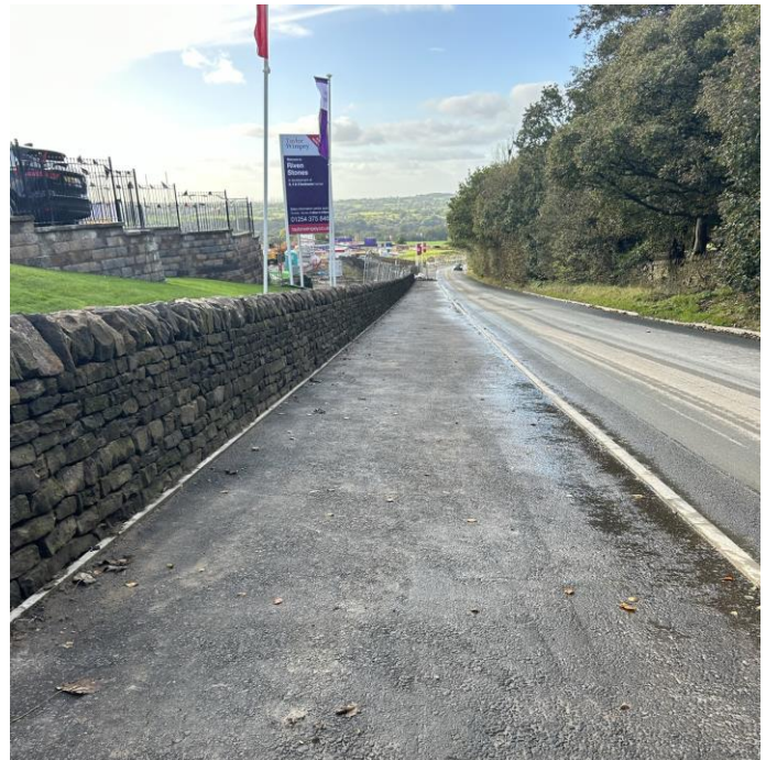
A new site access and footway with street lighting have been created as part of s278 works for the Taylor Wimpey/Barratt Homes development at Brokenstone Road, Blackburn
