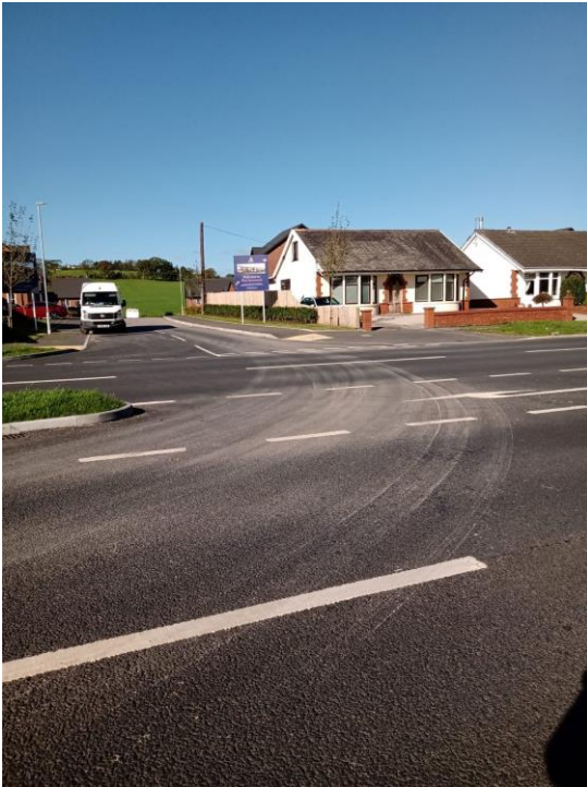
A new site access has been created through s278 works at Ramsgreave Drive, Blackburn
